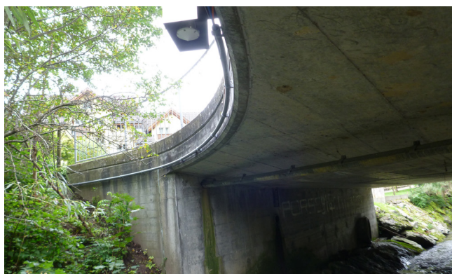
Figure 2: The gauge radar is mounted on the bridge, the pressure probe at the river bed.
