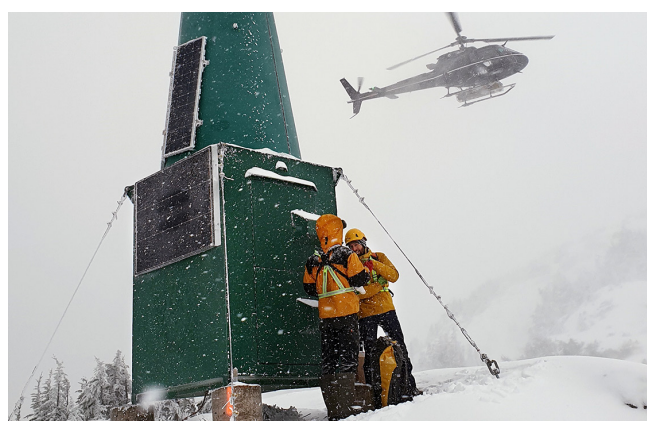
Figure 2: Mt Johnson repeater station: The region is characterized by harsh weather conditions that pose a challenge to installation and system operation.
