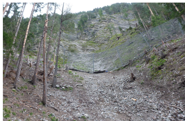
Figure 4: The construction site is threatened by two main gullies. Multiple lines of protection netting are designed to keep rocks from reaching the valley bottom.
