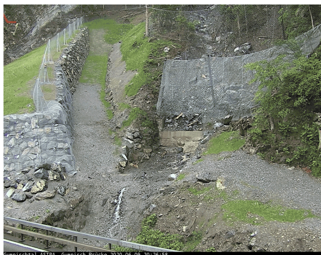
Figure 4 : Filets de protection.
